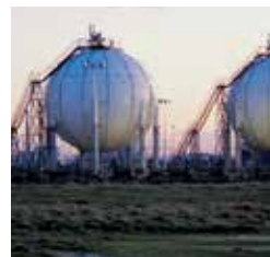
Oil & Gas Transportation & Storage
