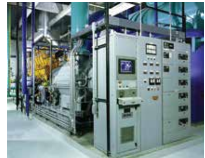
District cooling, U.S.
