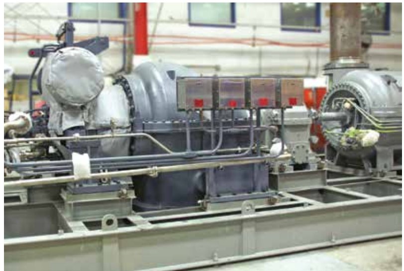
Steam Turbine Driving M Compressor
