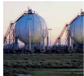
Oil & Gas Transportation & Storage
