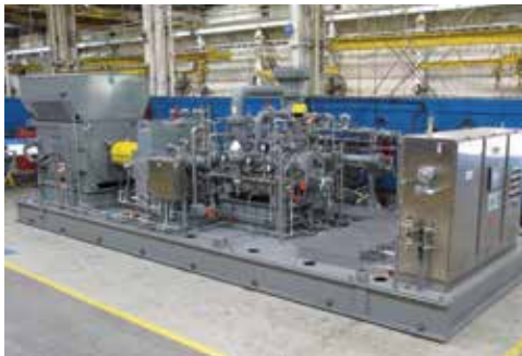
Gas processing, Trinidad
