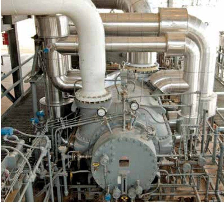
4,000-hp driveline in gas-processing application
