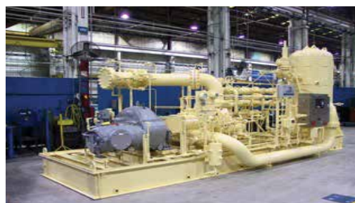
Steam turbine-driven driveline, Indonesia
