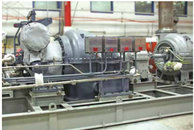
Steam Turbine Driving M Compressor
