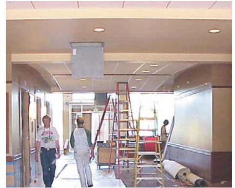
The building was constructed with people in mind. Increased ventilation, carbon dioxide monitoring and thermal control will lead to improved comfort.
