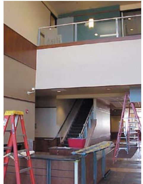
Cutting-edge technology will provide energy savings of 57% compared to a typical office building.
