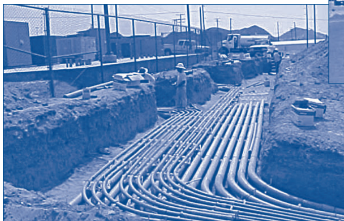
The project included a 7,200-square-foot turbine hall, a 3-mile high-pressure natural gas fuel line, and connections to the electrical substation feeding critical base electricity loads.
