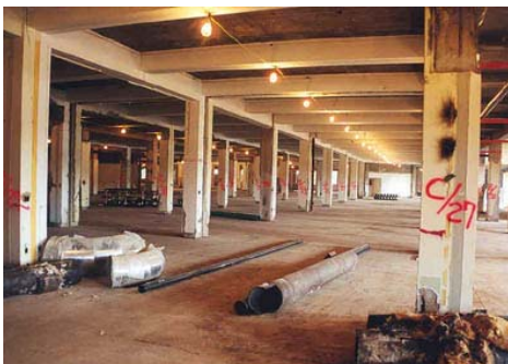
During the demolition and abatement program, everything was removed from Wedge 1, with 70% of the 83 million pounds of debris recycled.
