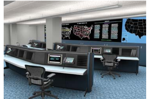
The Building Operations Command Center (BOCC) is a sophisticated, wall-to-wall monitoring system with around-the-clock personnel overseeing all building functions.
