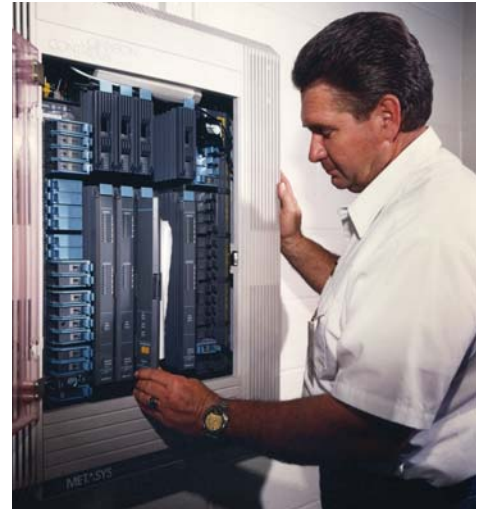
Matt Thomas, chief mechanical technician, examines a Metasys control panel.
