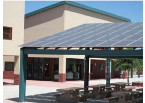
Norman N. Glick Middle School, Modesto, California uses photovoltaic panels to help meet the school's electrical demand, while providing a comfortable shaded break area for students.
