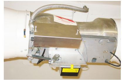
Actuator and UVM-1000 Installed
