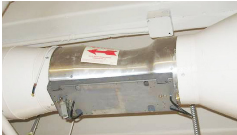
Actuator and Linkage Removed
