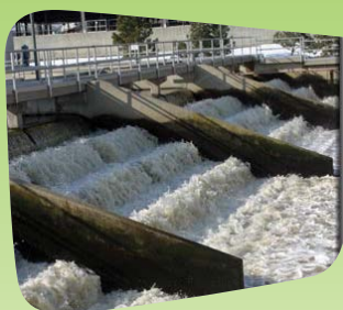
Back River Wastewater Treatment Plant
