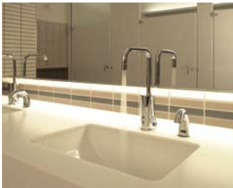
Low flow fixtures and dual-flush toilets significantly reduce water use across the campus. Harvested rain water is used to flush most of the toilets on the campus.
