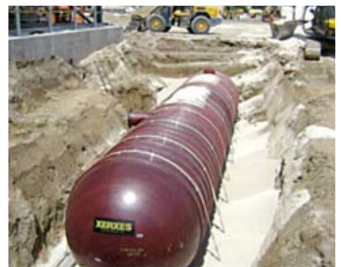
By capturing rainwater and snowmelt in this cistern, then cleaning and reusing it, municipal water use is reduced by 77 percent.
