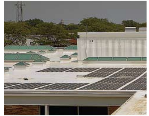
More than 14,000 square feet of thin-film PV cells are laminated to the roofing membrane of one building to generate electricity.
