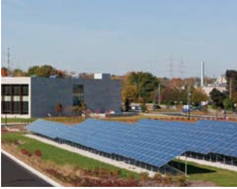
On the grounds, 1,452 solar photovoltaic panels make up one of the largest arrays in Wisconsin, delivering up to 250kW of electricity to the site.
