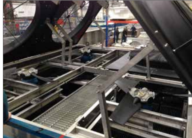
Figure 2 - Hinged Fan Panels and Interior Walkway
