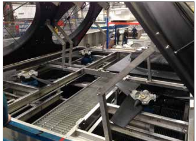
Figure 18 - Open Fan Panels on Top of the Unit
