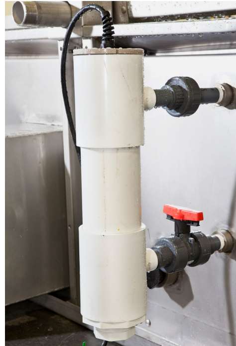
Figure 5. EWLC External Standpipe
